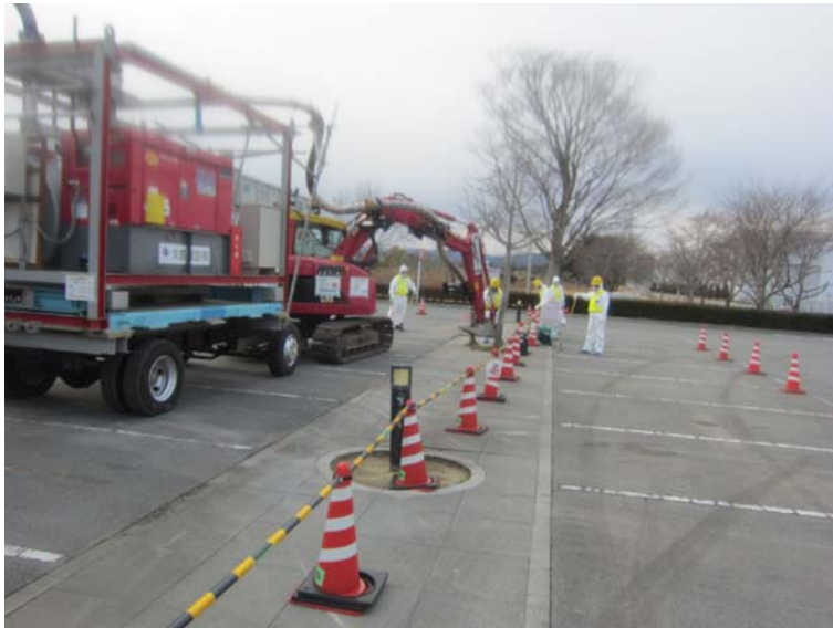
②-7 Collection work of dust and small debris at parking area of Main Anti-earthquake Building
