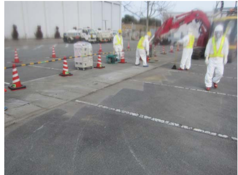
②-9 Collection work of dust and small debris at parking area of Main Anti-earthquake Building (after work)
