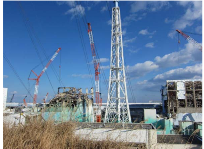
⑭— 2 Unit 3 Reactor Building Jan. 14, 2012 photo by TEPCO staff
