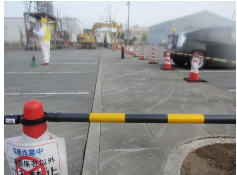
②-8 Collection work of dust and small debris at parking area of Main Anti-earthquake Building (after work)
