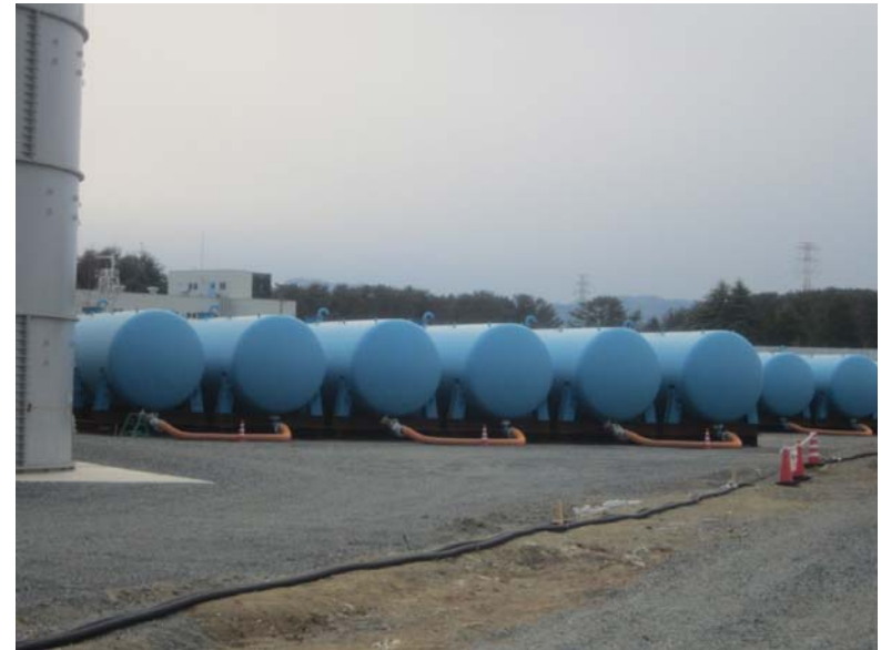
⑧-2 Tank array at H area Jan. 9, 2012 photo by TEPCO staff
