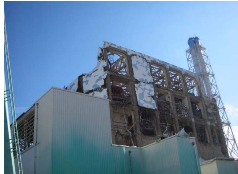
①-4 Unit 4 Reactor Building Jan.10, 2012 photo by TEPCO staff
