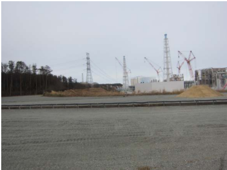
④-3 Look into Reactor Building from the hill in the southern side of Unit 4 Jan. 9, 2012 photo by TEPCO staff
