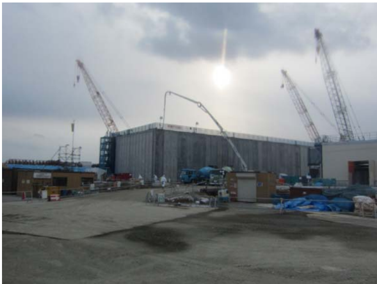
⑥-2 Waste sludge storage facility Jan. 9, 2012 photo by TEPCO staff
