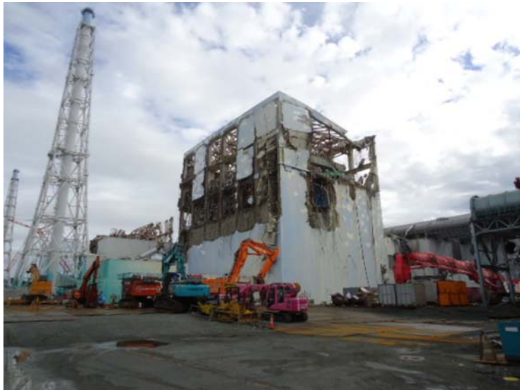
①-7 Removal of debris on the upper side of Unit 4 Reactor Building (before work)
