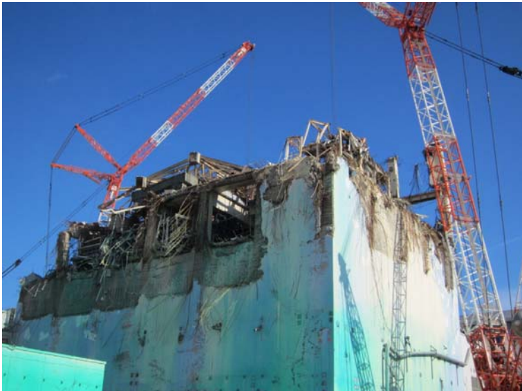
①-3 Unit 3 Reactor Building Jan.10, 2012 photo by TEPCO staff
