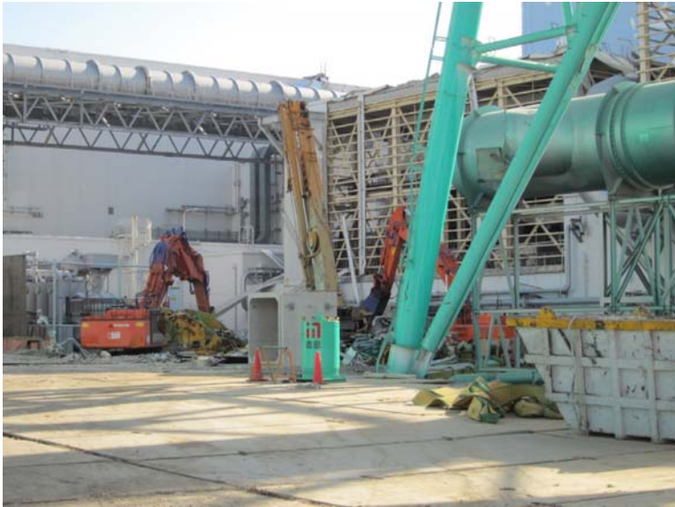
①-1 Removal of debris around Unit 3,4 Reactor Building Jan.10, 2012 photo by TEPCO staff
